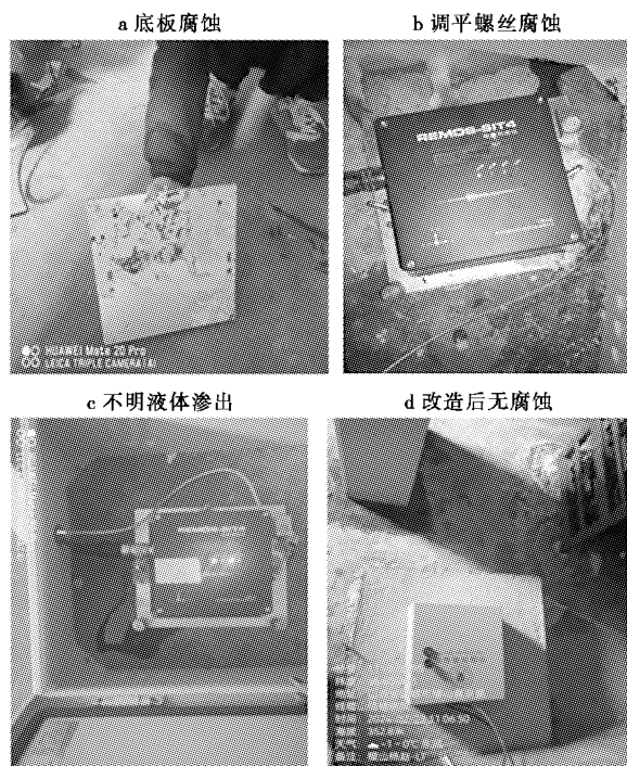
图4 运城站基本二类站烈度计衬板腐蚀与改造后情况 Fig.4 Corrosion of intensity gauge lining plate at Yuncheng Station basic class II station and the situation after renovation
